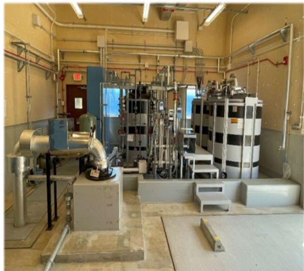
Figure 2: Sodium Hypochlorite & Fluoride Tanks
